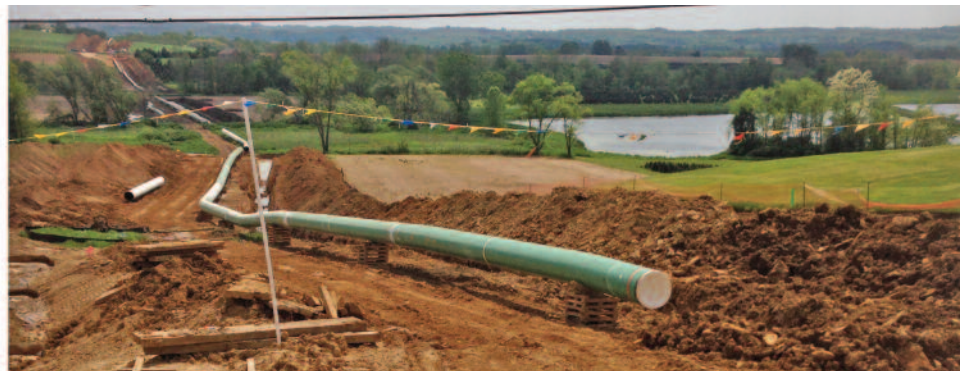
A SECTION OF THE ROVER pipeline construction near Shreve is shown in this photo taken May 17 by Randy Carmel. Hundreds of landowners are affected by the natural gas line that will stretch diagonally across Ohio for more than 700 miles.
